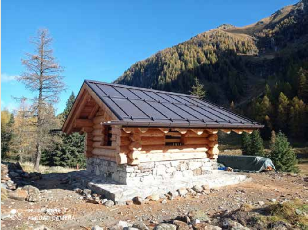
Figure E – Shelter in the process of construction by Primiero UDF at Socede di Sopra, Castello Tesino. Work will be completed in 2023. (M. Zotta, APT Forestry Department Archives)
