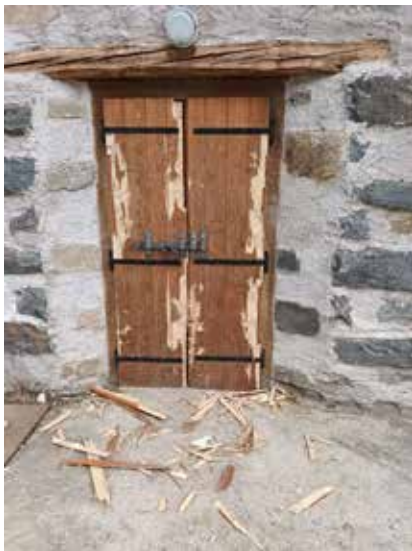
Photo 15 – Door damaged by a bear in Val Giudicarie (V. Calvetti, APT Wildlife Department Archives)
