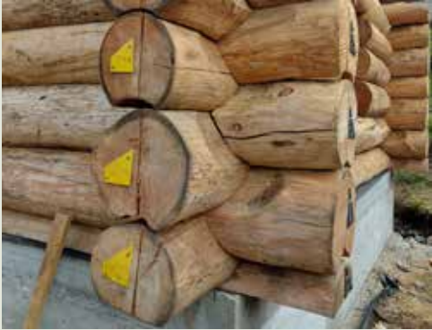
Figure A – Detail of corner joints used in the construction of the shelter at “Sette Laghi”, Torcegno. (S. Liberi, APT Forestry Department Archives)
