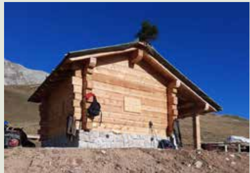
Figure D – Shelter in the process of construction by Tione FDO at Fontanelle-Prada, San Lorenzo Dorsino. Work will be completed in 2023. (G. Antolini, APT Forestry Department Archives)
